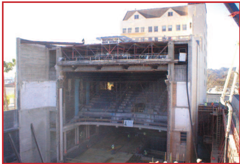
Top left: The theatre in the old days. Top right and above: The stage house renovation.
